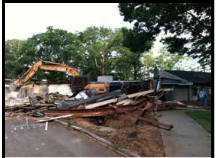
AYC Clubhouse was taken down and is under construction. Look for an updated photo of the rebuild in the next Flyer!
